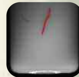
Side walls cracks control
