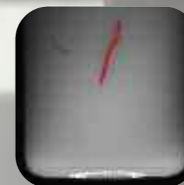
Side walls cracks control
